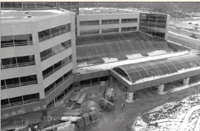
Images show construction of the Pomerantz Family Pavilion in 1996 where the main eye clinic is located.
